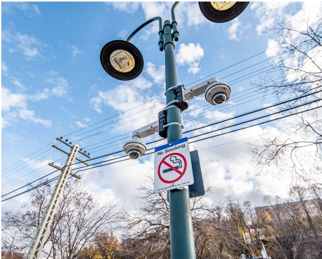
DESIGN AND CONSTRUCTION SERVICES FOR SECURITY, AUDIO-VISUAL AND FACILITY ENHANCEMENTS AT VARIOUS METRO-NORTH STATIONS MASS. ELECTRIC CONSTRUCTION CO. VIEW: TRACKS 1 & 3 - CAMERAS INSTALLED > NE PHOTO: 13241.008.005 DATE: 11/25/2020
