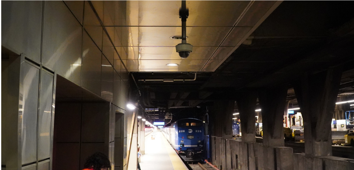
Security systems help safeguard Metro-North's infrastructure, operations, customers, and employees.
