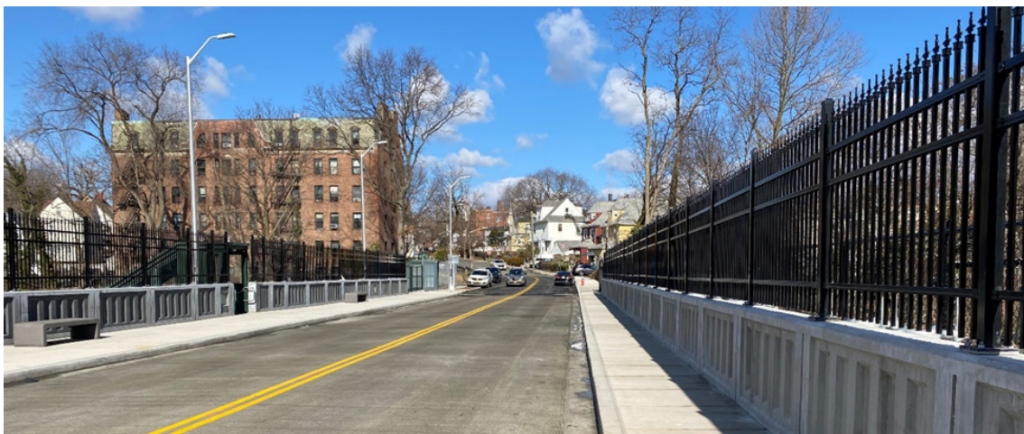
Bridge replacements in Mt. Vernon over the Metro-North New Haven Line were completed ahead of schedule.
