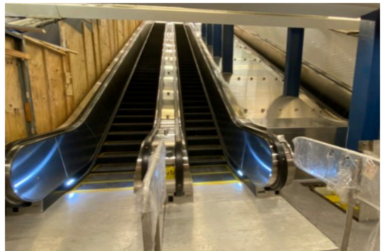
All three escalators are now back in service
