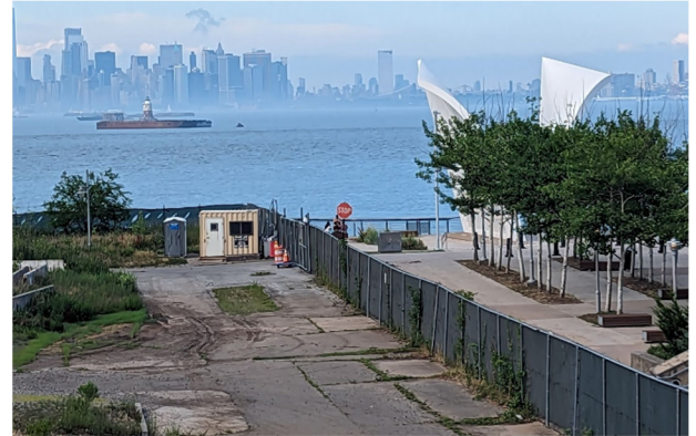
View northeast of construction fencing at the former New York Wheel Garage site
