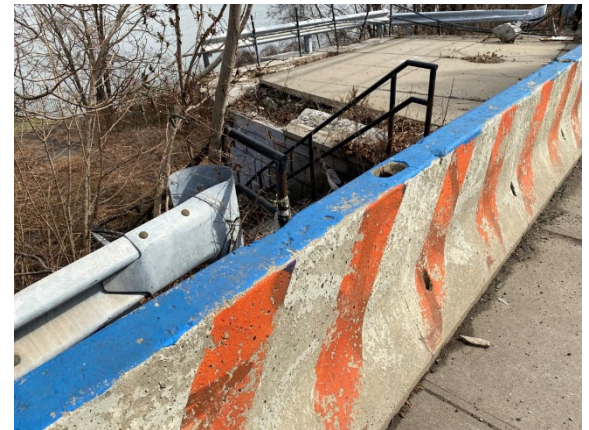
Overlook north of Richmond Terrace; which is blocked from pedestrian access due to its state of disrepair.
