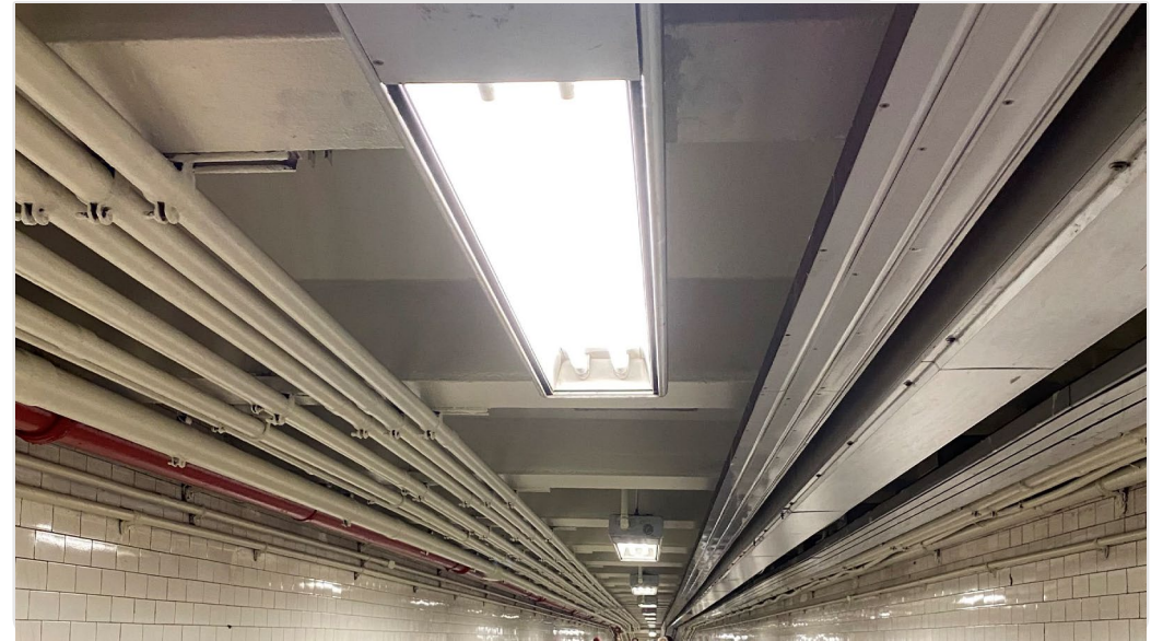
Example: New, brighter LED installed at York St Station
