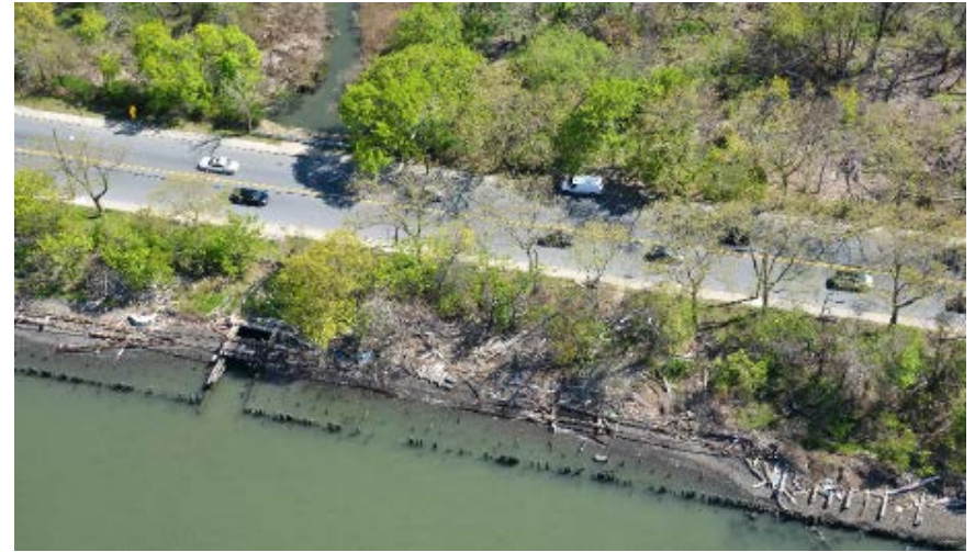
At-Grade: View of ROW and destabilized shoreline near Snug Harbor
